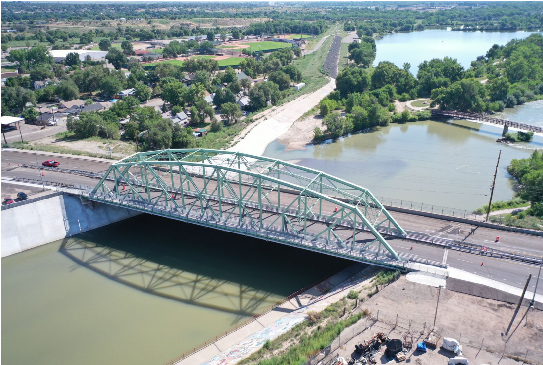
Completed Complex Truss Bridge Rehabilitation (US50 BUS over the Arkansas River - K-18-L)
